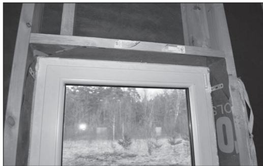
Figure 5. The assembly of the window element in the house frame construction with the made by workers of the analyzed enterprise.
